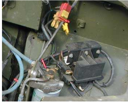
Figure 4: The left foot well, showing the relays and the fuel filter, the red and yellow relay are fan and starter respectively.
